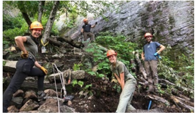
Conservation Team crews worked at the base of Thin Air Buttress of Cathedral Ledge in New Hampshire for several weeks, removing rotten timber structures and replacing them with a sustainable stone staircase that will last. Ancestral lands of Wabanaki Confederacy, Abenaki/Abénaquis, and Pequawket. © Cait Bourgault
