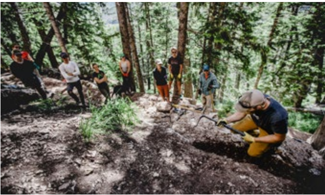
A Conservation Team crew member demonstrates a technique for creating the foundation for a stone retaining wall structure in Ten Sleep Canyon. Ancestral lands of Crow, Cheyenne, and Sioux. © Kris Ugarriza
