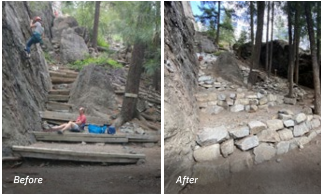
This belay area at Fun Rock in Washington was supported by a set of rotting timbers, installed decades ago, which were collapsing and destabilizing the hillside. These new stone steps reinforce the hillside, protect the trees, and give climbers a sustainable area to belay without damaging the surrounding environment. Ancestral lands of Okanagan and Nlaka'pamux.
